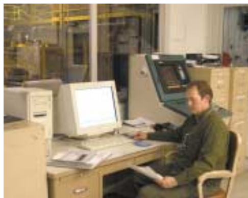
Plant manager Don Ball using the SCADA computer system to monitor all aspects of the plant's equipment operation and performance.
